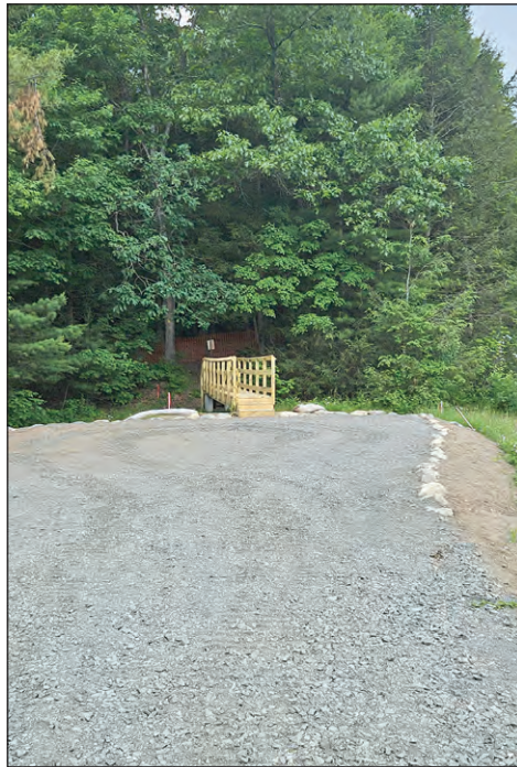
A gravel path leads to and from the bridge at Lithia Springs.
